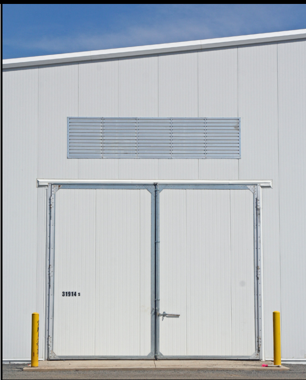
Figure 2.9. Exhaust louvers above access doors.
