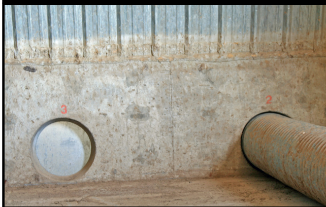
Figure 2.6. Ventilation duct openings from plenum chamber.
