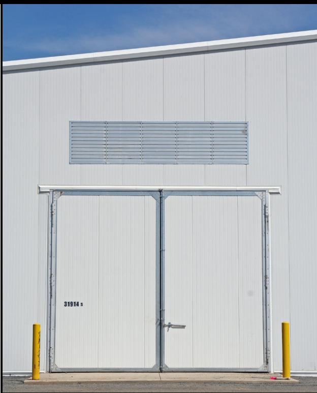
Figure 2.9. Exhaust louvers above access doors.
