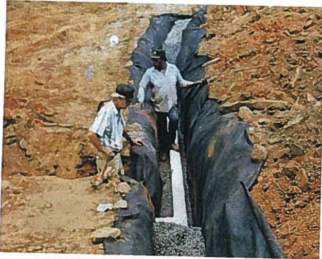
Figure 10D-28 Perforated collector pipe installed the gravel envelope with trench lined with geotextile
